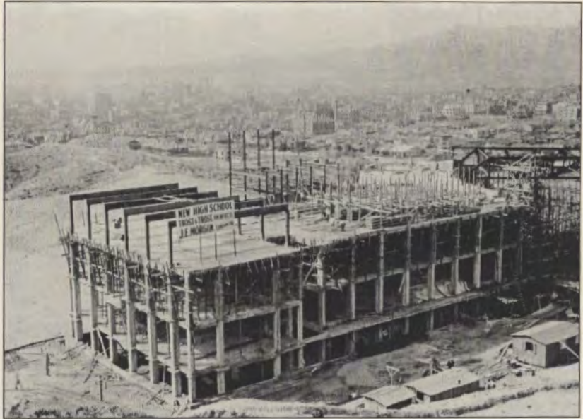
El Paso High School under construction in 1915. Courtesy of the University of Texas at El Paso Library, Special Collections Department, J.E. Morgan & Sons photographs, PH020.
