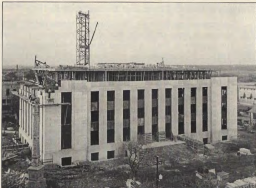
The Grayson County Courthouse under construction in 1935. Courtesy of the University of Texas at El Paso Library, Special Collections Department, J.E. Morgan & Sons photographs, PH020.
