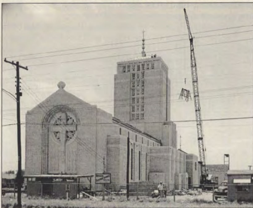
Christ the King Church in Dallas in 1956. The Dallas branch of J.E. Morgan & Sons helped keep the firm profitable after World War II. Courtesy of the University of Texas at El Paso Library, Special Collections Department, J.E. Morgan & Sons photographs, PH020.
