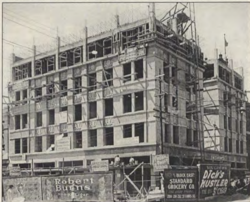
The Banner Building under construction in 1910-1911. Signs for "Sorenson & Morgan, General Contractors" and "Trost & Trost, Architects" are visible on the building. Courtesy of the University of Texas at El Paso Library, Special Collections Department, J.E. Morgan & Sons photographs, PH020.
