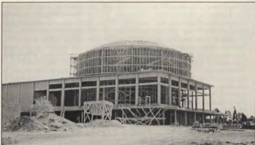
Temple Emanuel under construction in Dallas in 1957. J.E. Morgan & Sons possessed the technical expertise to construct unusual and difficult designs, such as this round dome. Courtesy of the University of Texas at El Paso Library, Special Collections Department, J.E. Morgan & Sons photographs, PH020.
